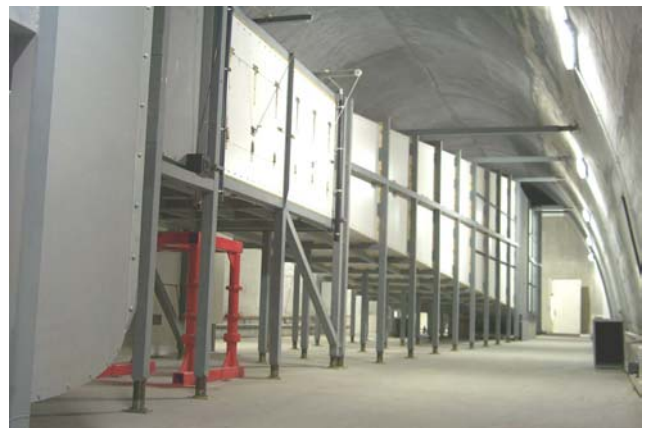
Fig. 13 : CMEFE main wind tunnel, 300 kph, 6.6 ft x 4.9 ft
